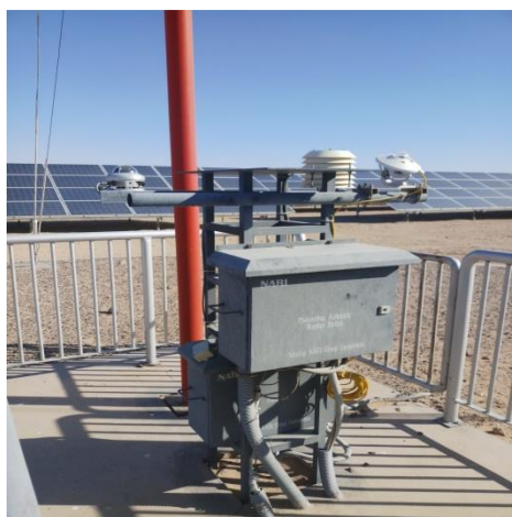
Figure2.Meteorological station of Adrar solar power plant.
