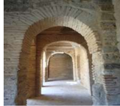
Picture : Overreaching Broken Arch above the Door Connecting the First and Second Wings
