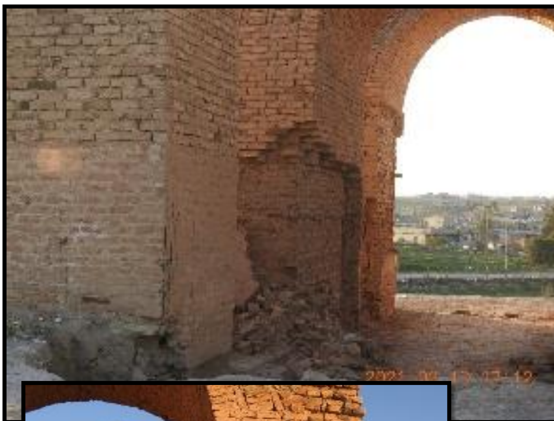
Tabira Gate after the bombing And maintenance of the second contract It is clear from the picture that the maintenance has not ended The photo was taken on February 13, 2021
