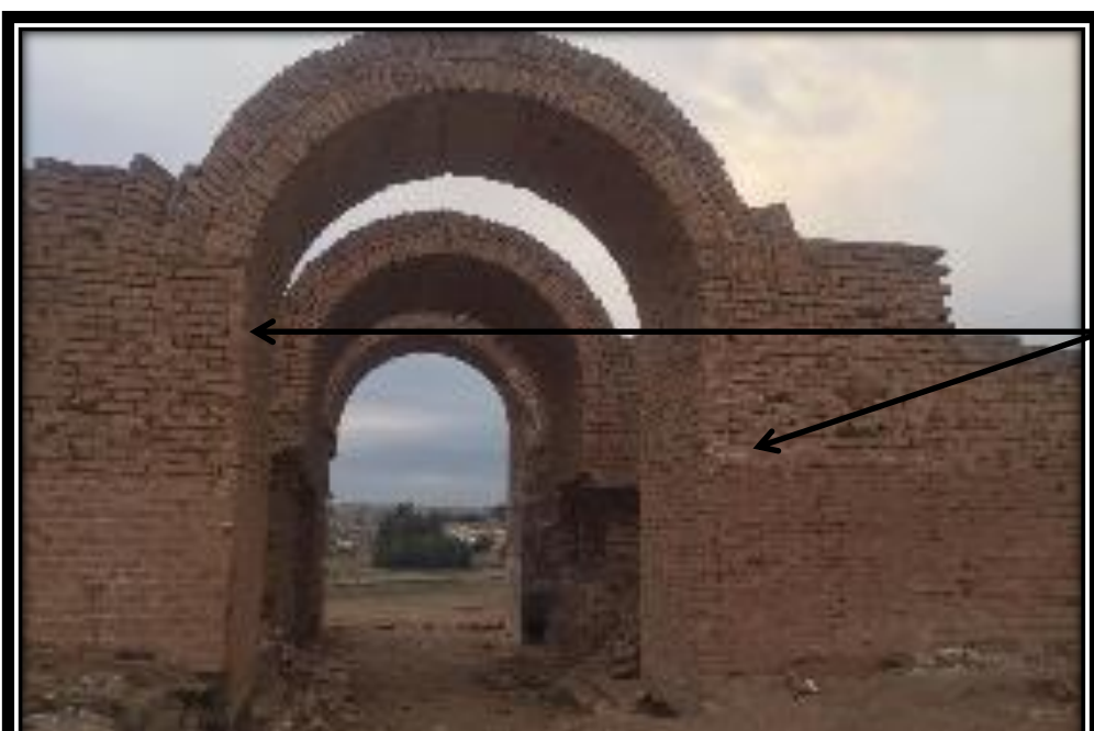
Third arc It is clear that was not damaged
