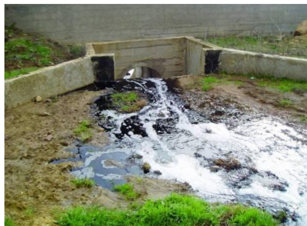
Figure 4. Leachate leaving the landfill (after 3rd lagoon).
