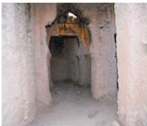
Picture N° (08): Supporting system.
