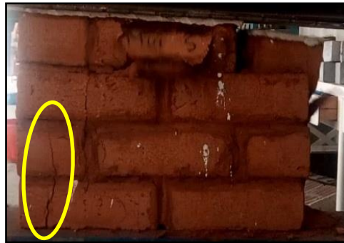
Fig. 12 – Rupture of the wallets type C: Obtaining of the first fissure at t=26s ; Rupture of the wallets at t=63s .
