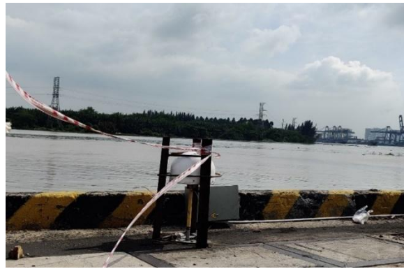
Fig. 4 – Location of Real-Time GNSS monitoring point at the target wharf
