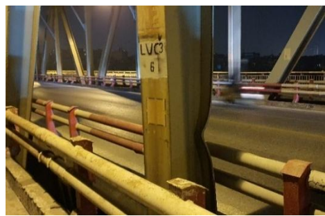
(b) Local imperfection at the truss of the Chuong Duong bridge
