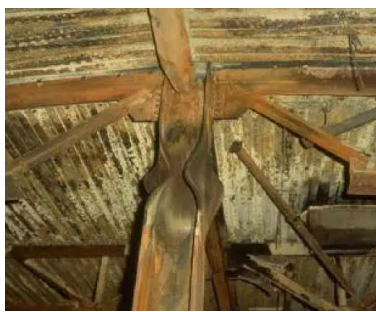
(a) Local imperfection in steel columns [1]
