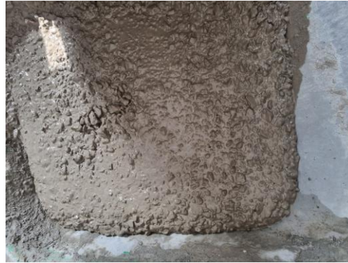
Fig.9 -Segregated concrete in MIX I
