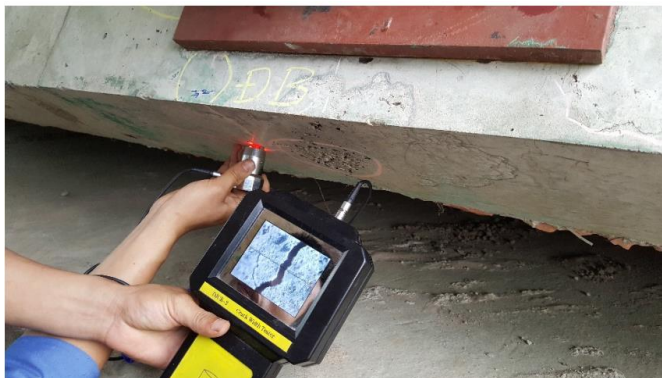
a) Cracks at the lower end of Strut 3
