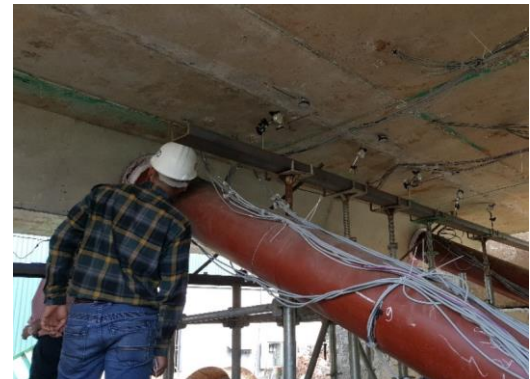
b) Monitoring cracks at the upper end of Strut 3
