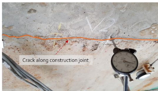
a) Cracks occurred at the construction joint at an applied load of 52 kN
