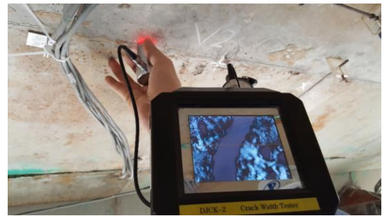
b) Monitoring crack opening during the test
