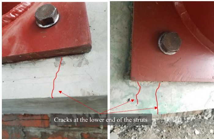
Fig. 6 - Cracks at the lower end of the struts during fabrication
