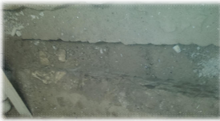
Image (03): Traces of drainage channels inside the mosque.
