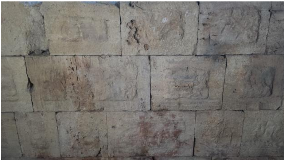
Image (05): Protrusions on the wall.
