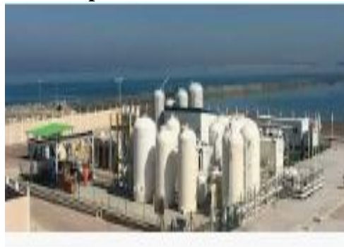
Figure (05): Ghantoot Experimental Water Desalination Plant
